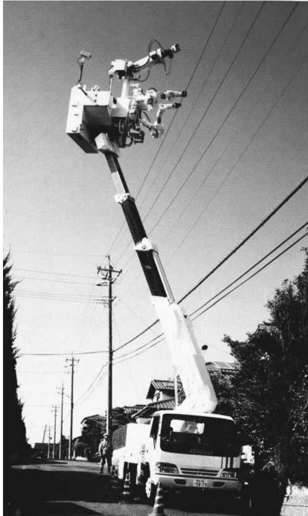
Figures 14.1–14.3. Telerobotic system for repairing high-voltage power lines. Kyushu Electric Power Co. Allows a human operator to safely repair high-voltage electrical power lines. Thirteen of these systems have been deployed in Japan to repair high voltage power lines without service interruption. These systems have both teleoperator and telerobotic features.
